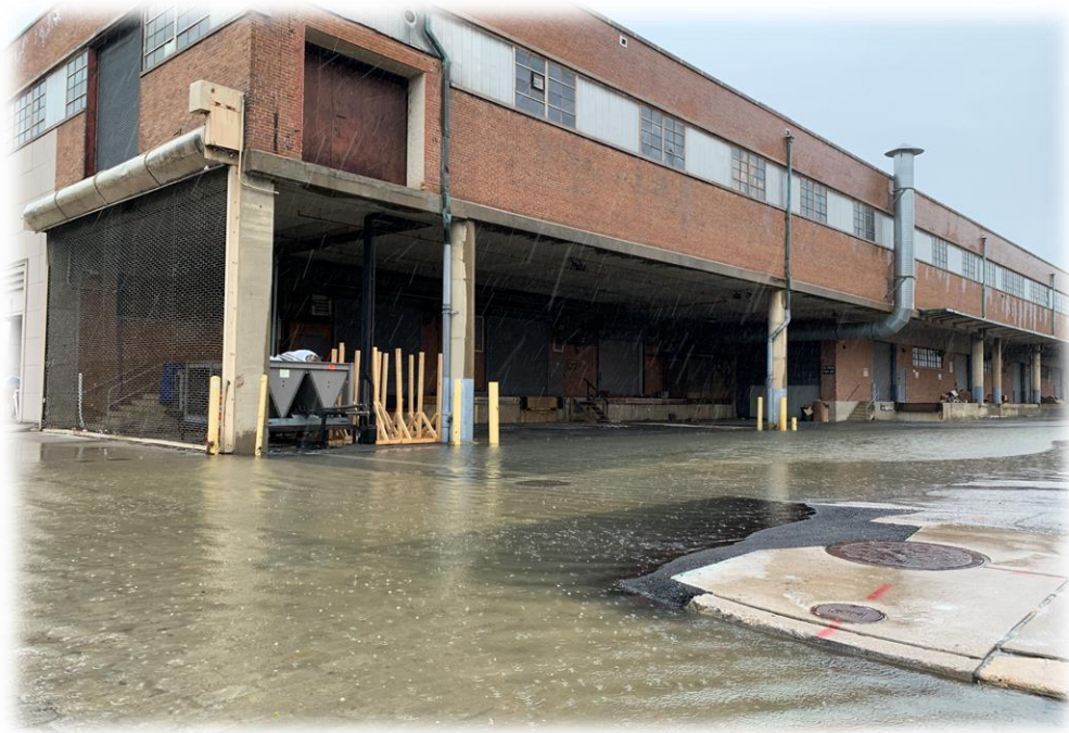
Figure 25: Nuisance flooding in Fells Point in May 2020. The northwest branch Patapsco River tidal gauge registered a 4.3 feet tide high during this period
